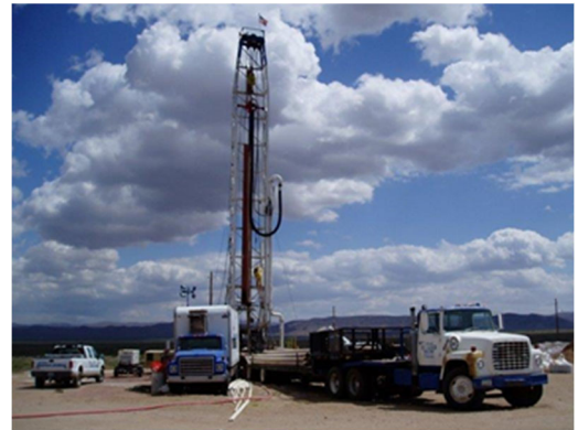
Two to three drilling rigs were running simultaneously for over a year
