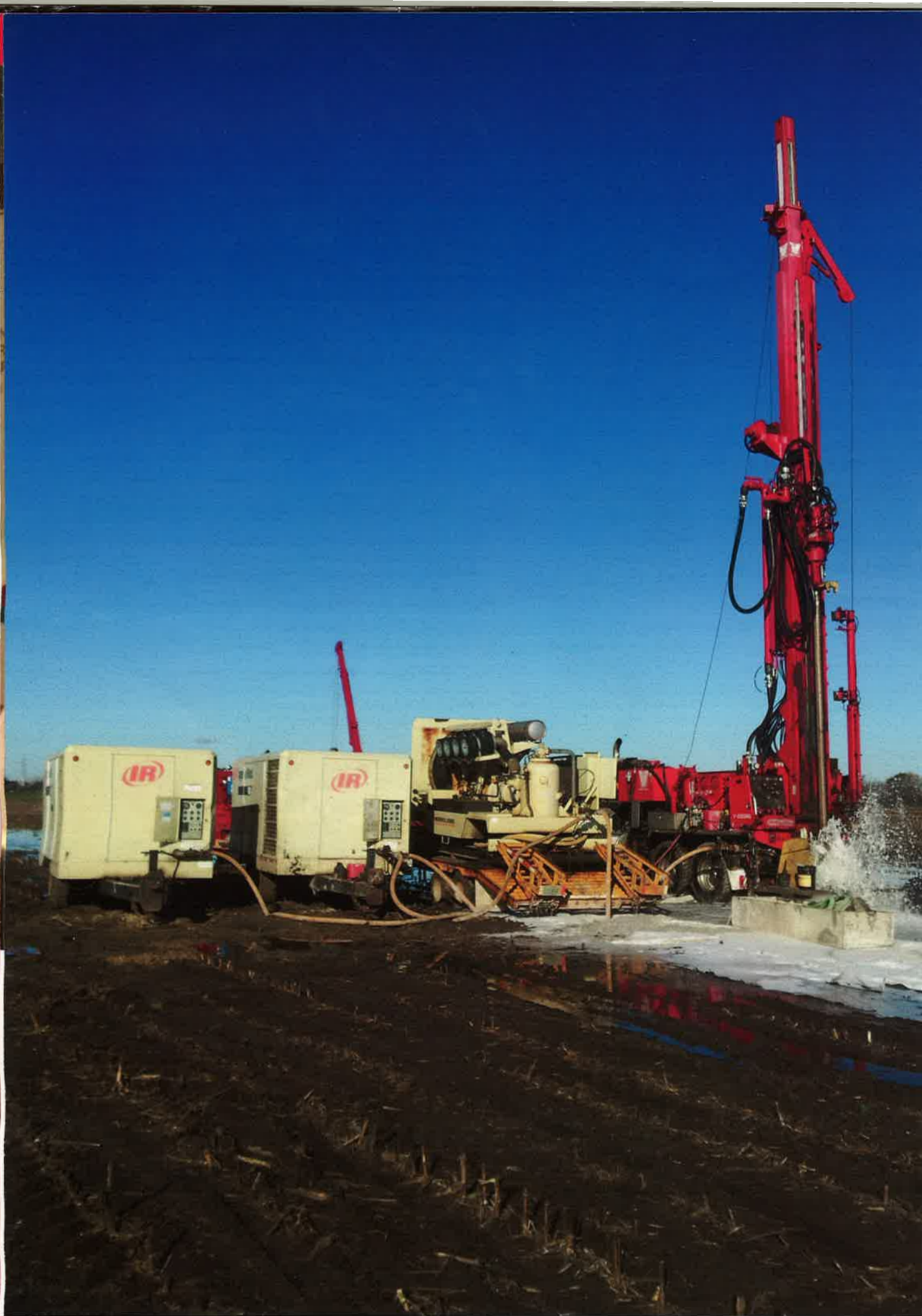
"The Art of the Water Well" deals more with higher capacity wells, like those for large-scale irrigation or municipal use. But some of the advice, particularly about communication, can smooth out work at any jobsite. Source: Sam's Well Drilling / File Photo
